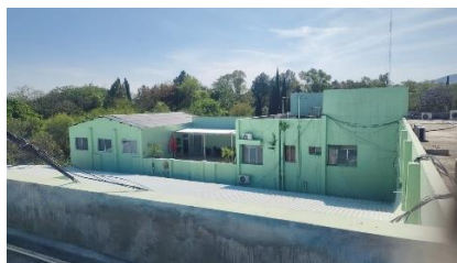
Cable Routing Towards Main Building – Ground Floor
