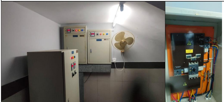
Control Room for East/West Buildings
